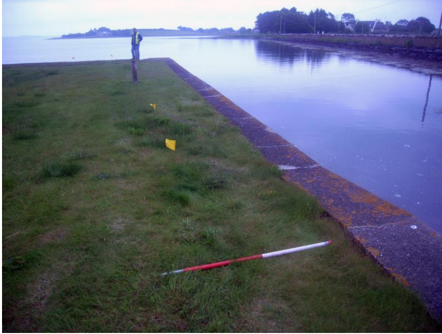
Figure 15: Partial collapse of southern wall of quay, indicated by change of levels in coping. Yellow flags indicate areas of collapse at surface level
