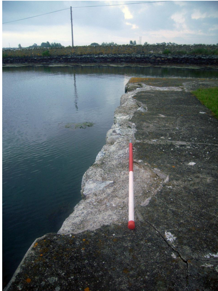
Figure 13: Modern damage to coping on north wall of quay
