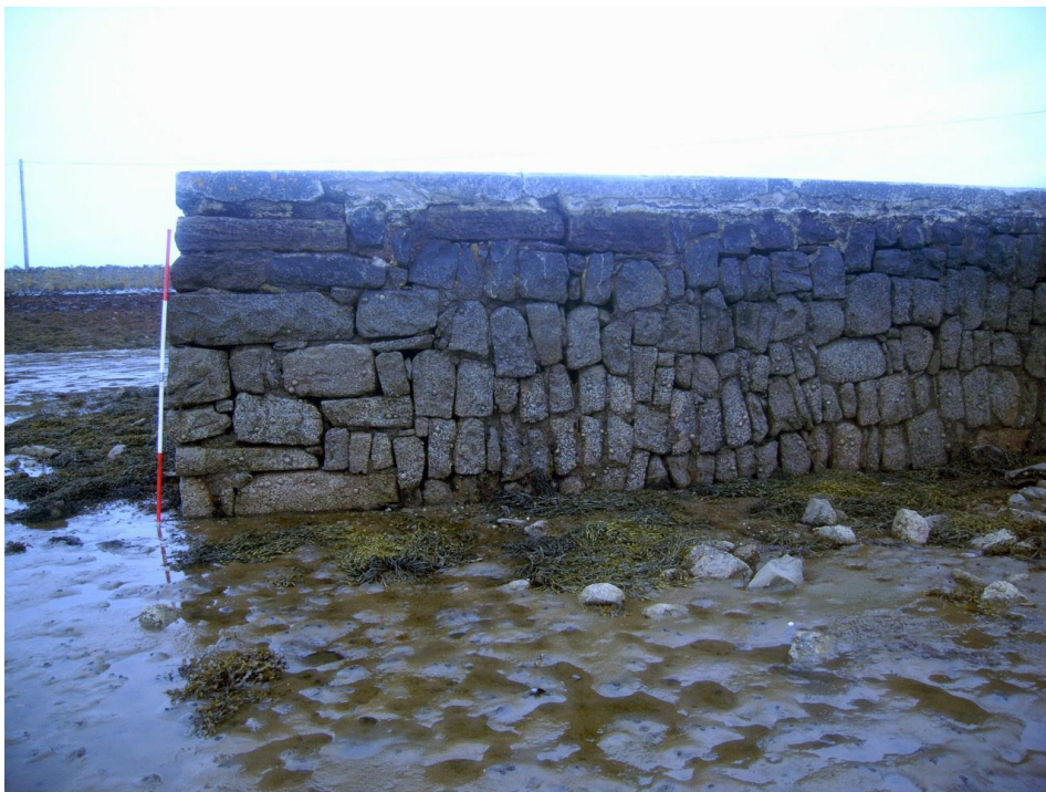
Figure 16: View of north-facing (seaward end) of the quay wall, showing construction materials and techniques
