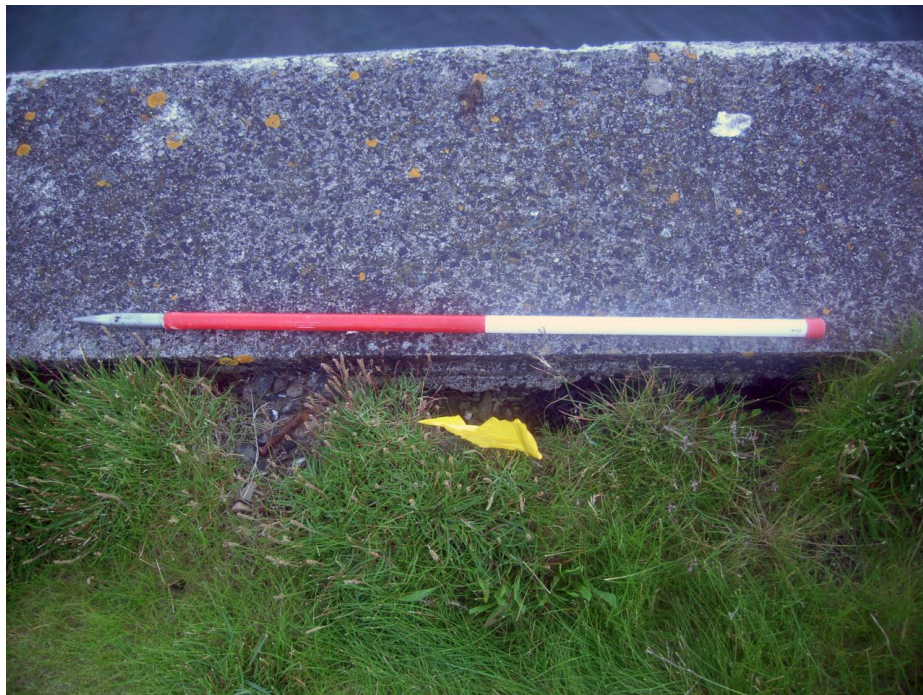
Figure 14: Portion of partial collapse of quay
