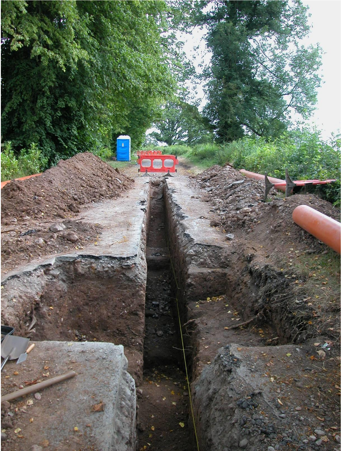
Plate One: General view of site showing pipe trench and the excavation trench, looking north-east. The NW trench is on the left hand side of the photo and the SE trench is on the right hand side
