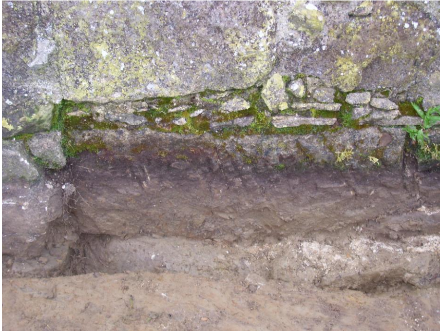
Plate 7: View of quoin stone with diagonal tool marks at base of northern castle wall (context 306) in Trench 3
