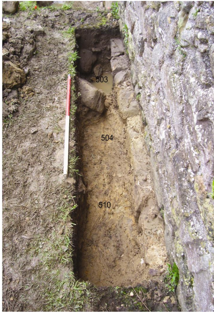
Plate 9: Post-excavation photograph of Trench 5 showing subsoil (context 510), foundation plinth (context 504) and excavated soakaway (context 503)
