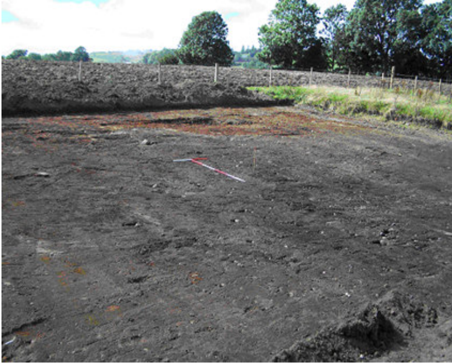
Plate 10 View of development site excavated to glacial subsoil level, showing the dark staining to northeast. Looking northwest.
