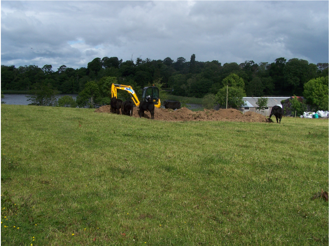
Plate Six: Mechanical topsoil stripping of the proposed application site, looking north-west with Marlaco Lough in the background
