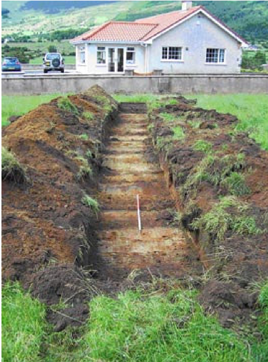
Plate One: Trench One following excavation to the surface of the subsoil (Context No. 103), looking west.
