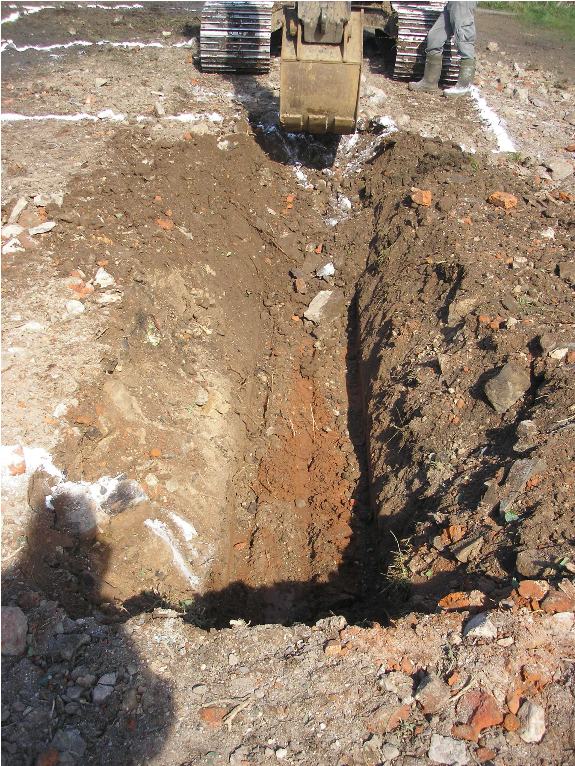
Plate 3: Excavation of the foundation trenches, showing mixed rubble deposit (Context No. 101) and the natural subsoil (Context No. 103), looking north.
