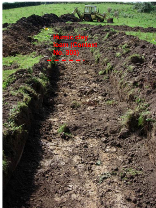
Figure Fifteen: Trench Three following excavation to subsoil (Context No. 308), looking west
