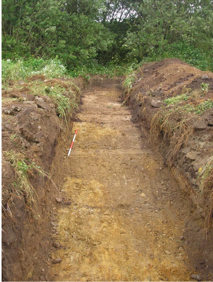
Plate Five: Trench Two following excavation to subsoil (Context No. 205), looking north
